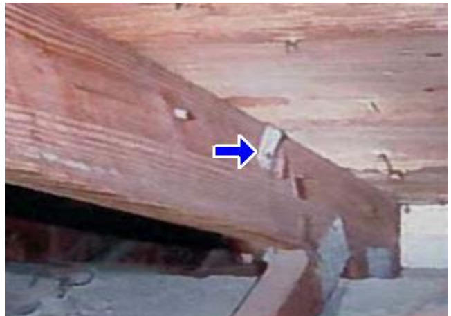
Roof to Wall Connection - Straps (Backside)
